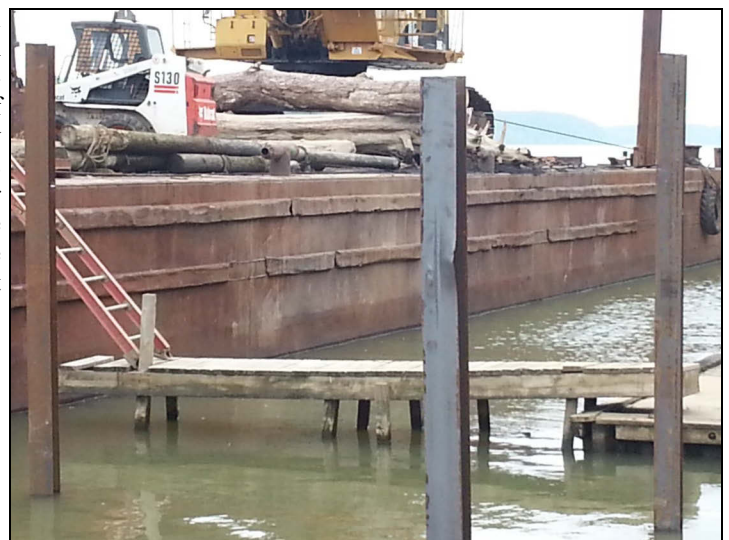
Looking upstream, installation equipment on barge in background; in foreground, new steel pilings for LSC committee boat will allow for significant river level fluctuation.
